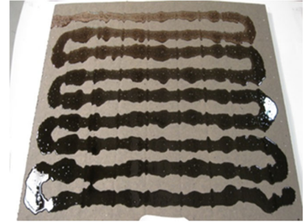
Freshly applied beads of XR Stick on mechanically attached Polyisocyanurate insulation board @ 4" o.c.
