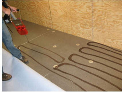
Bead application of XR Stick in cartridge on mechanically attached Polyisocyanurate insulation board @ 6" o.c.
